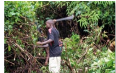
Clearing a field for construction of a CSIO Office in Grand Kru County
